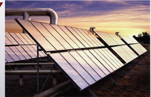
Solar thermal installations
